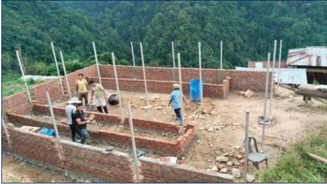
Figure 6: Snapshot of mushroom shed picture taken during the construction stage in May-June 2025
